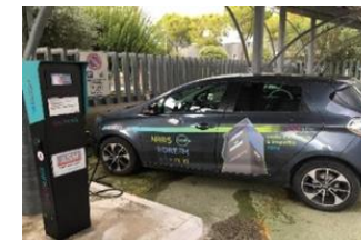
3 Smart Charging Stations
