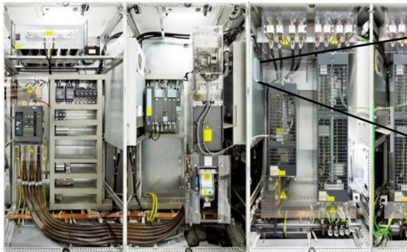
Combining the information from the IR-Camera and the magnetic field sensor to localize electric faults in power cabinets by deep learning methods
